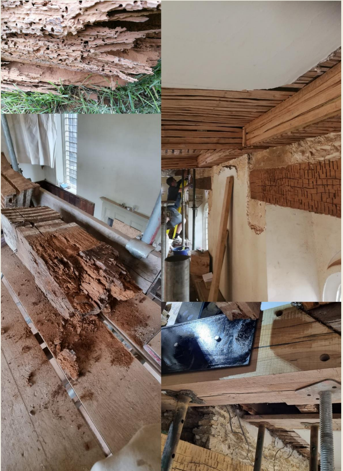
Above: Collage of views of damage and repairs in Corsham Almshouses
